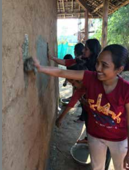
Students' learning a traditional wall treatment technique at Immersion Module at the Polo forest in Vijaynagar
